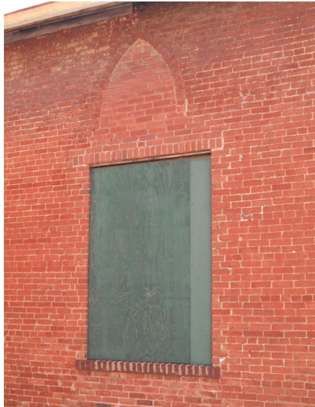
Remnants of the Gothic arched windows can still be seen.
